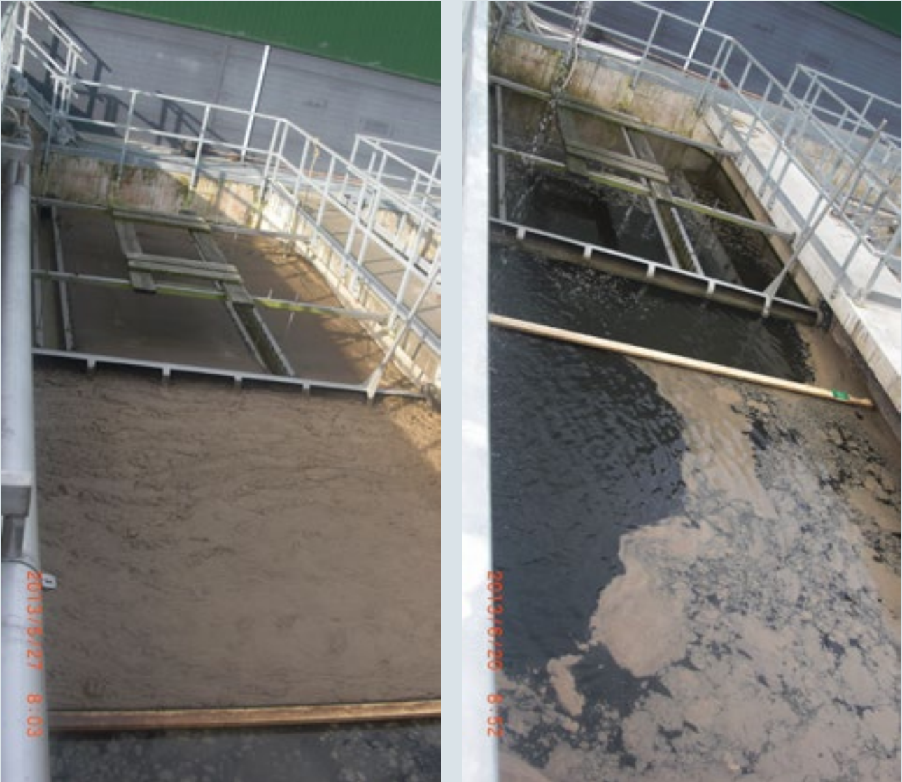
2 pic. Wastewater treatment plant before and during GREASOLUX use.
